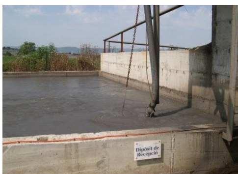
Picture D.1: Reception tank.
