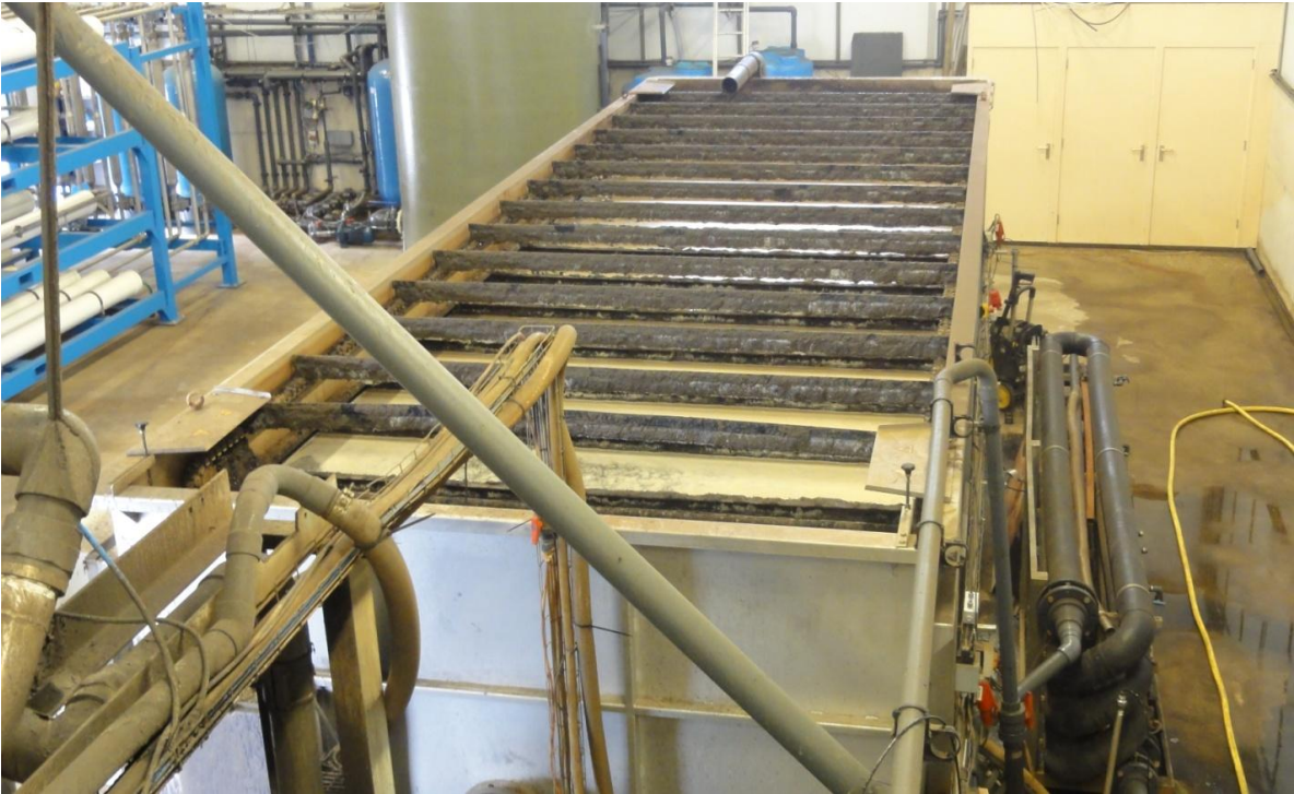
Picture C.7: Scrapers remove the flotation sludge from the flotation unit.
