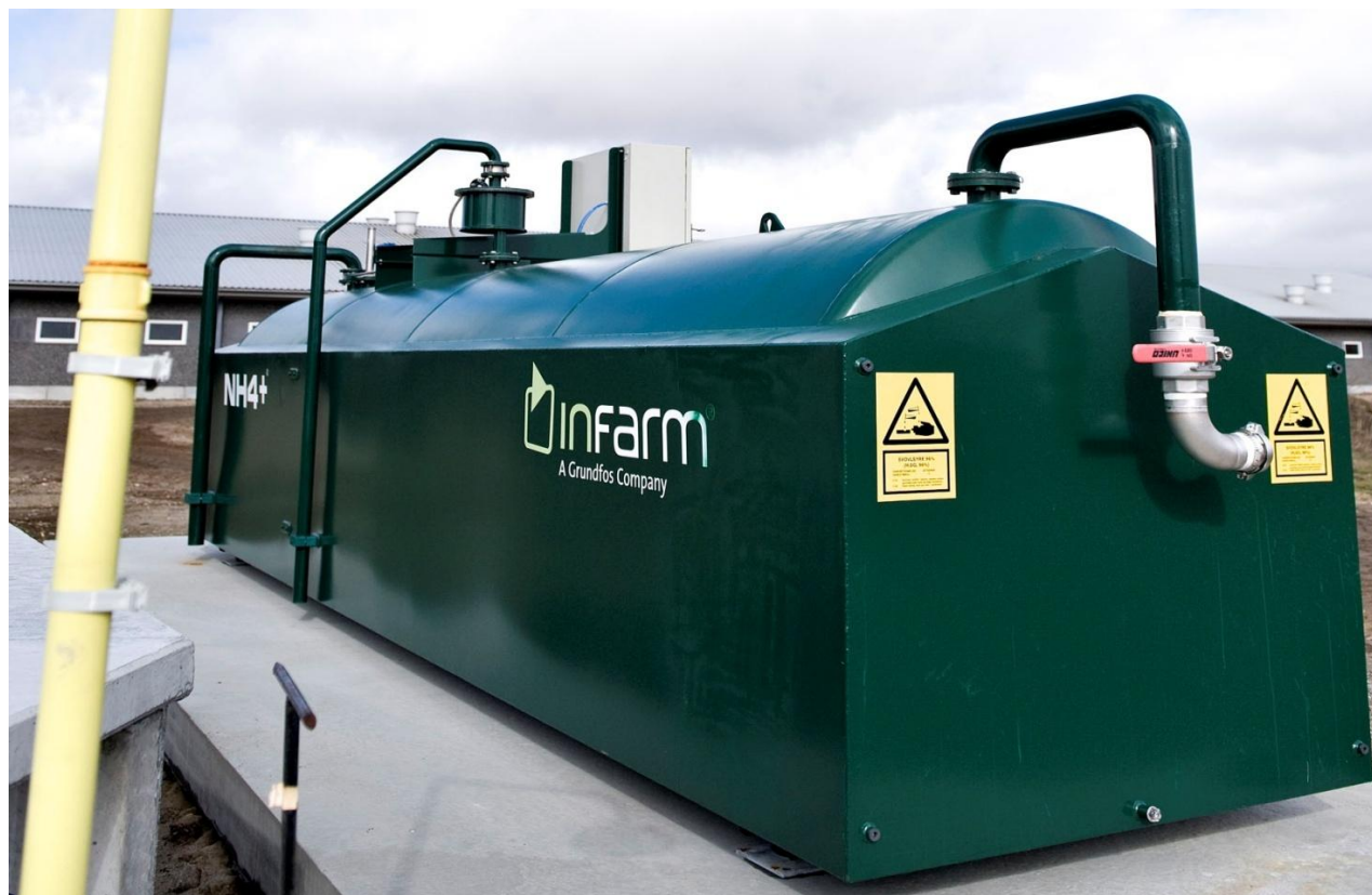
Picture B.1: Acid tank
