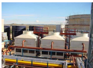
Picture E.10: Evaporative coolers
