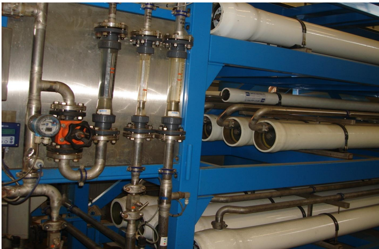
Picture C.9: Reverse osmosis unit.
