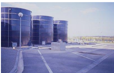
Picture E.1: Reception Tanks
