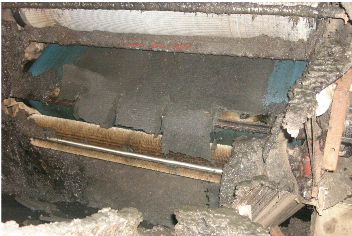
Picture C.5: Separation solids are scraped off the filter belt press.
