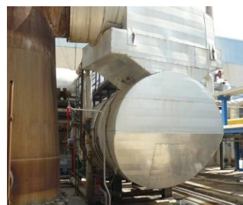
Picture E.9: Boiler (heat recovery)
