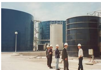
Picture E.2: Anaerobic digestion reactors
