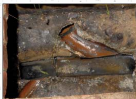
Figure 17. Material fire-damage around River opposite Maria Isid.
